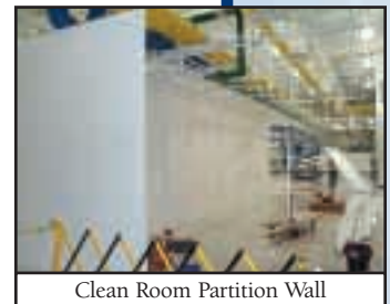
Clean Room Partition Wall
